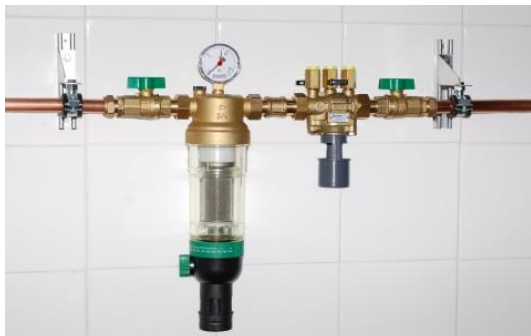
RPZ Option F and wall fixing brackets – providing rear clearance as required by the Water Regulations
